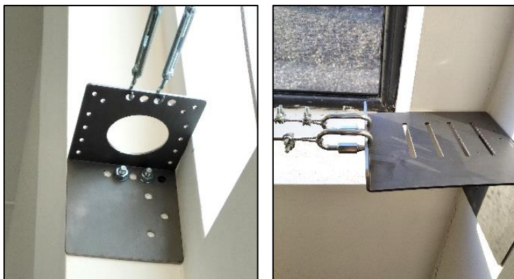
Figure 3. Steel wire with tensioners and the consoles on the wall
